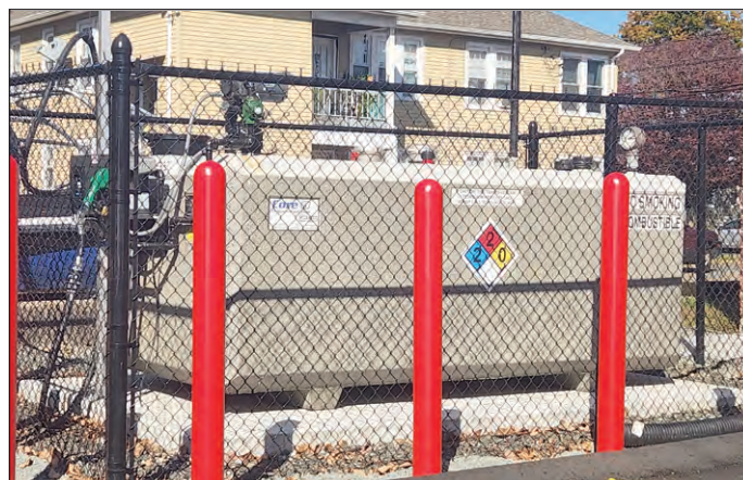
A shot of the new storage fuel tank at Station Five, part of the capital improvement projects for Station Five.
