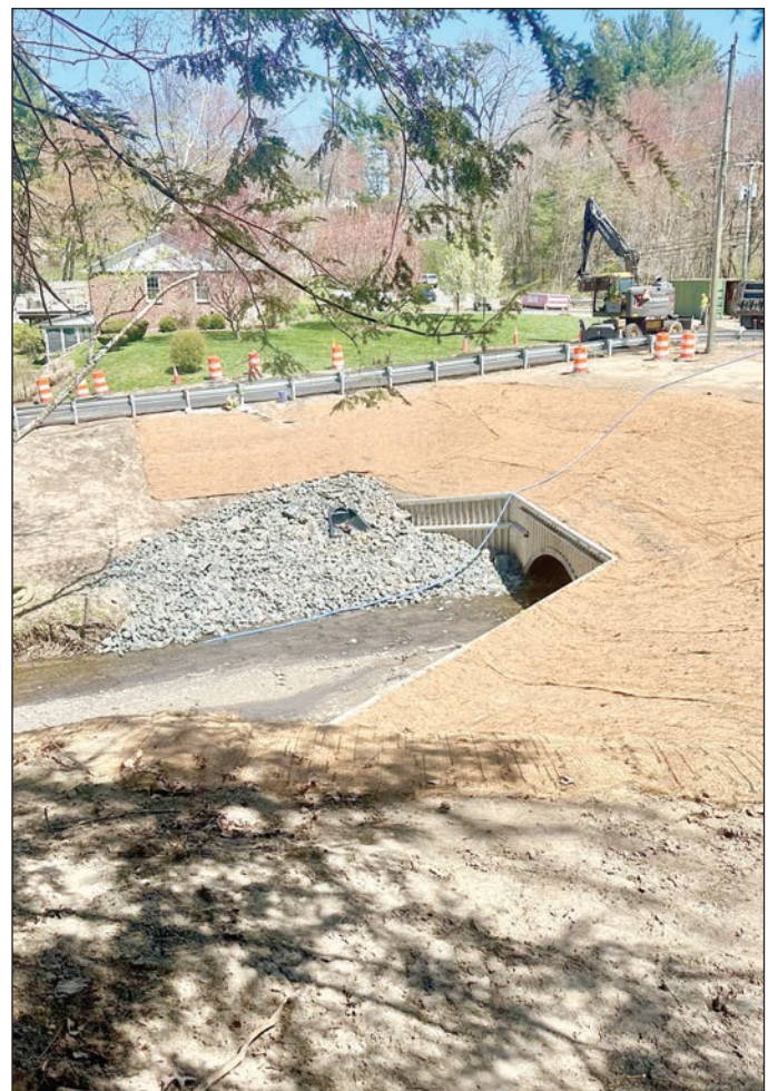
At last, North St. has re-opened to thru-traffic. A culvert was under repair since late last year. Materials delays caused the project completion to be pushed back several months. The repairs were finally completed at the end of April and the road was fully re-opened to all traffic last Friday afternoon. SUBMITTED PHOTO
