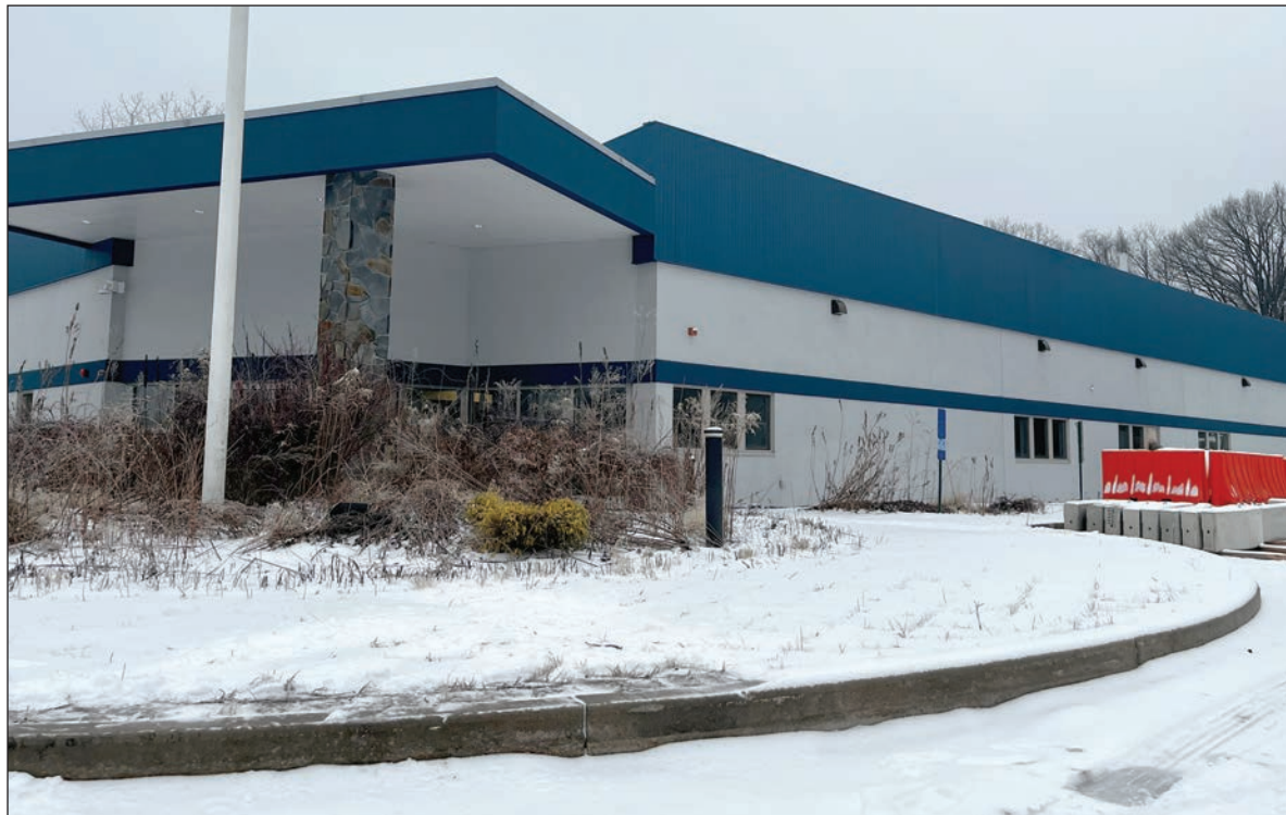
Construction is nearly complete on the new Agawam Police headquarters. It is scheduled to open in June.
