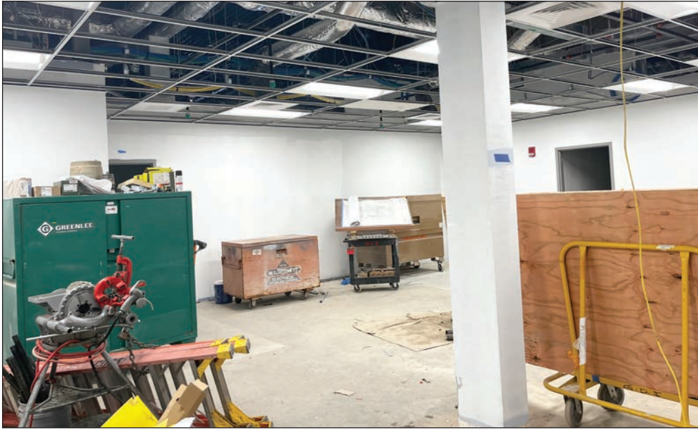
Significant progress has been made on the construction of the new police department headquarters.
