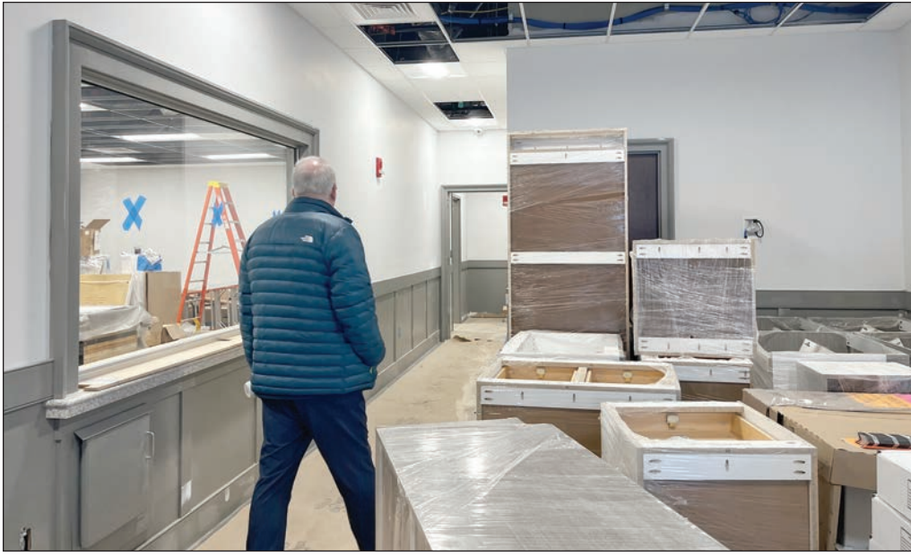
Right as people enter the new police department, they will see the records window to their right should they need to request something.
