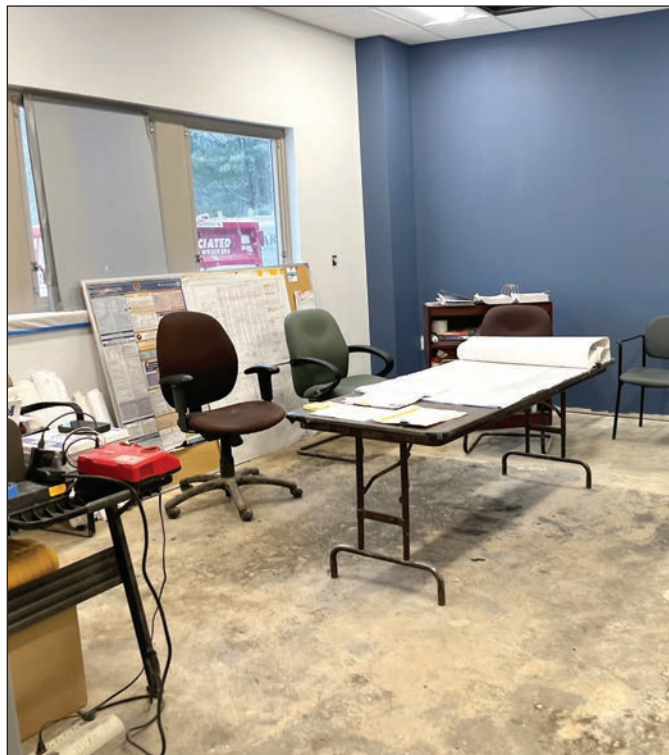
The new police chief's office is in good shape as the police department construction continues.
